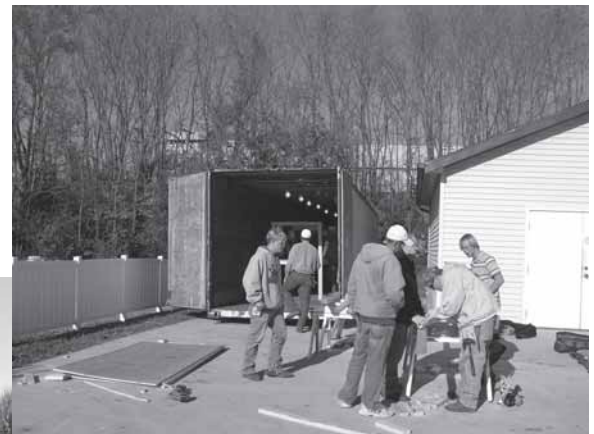
Students and instructors from Nichols Carrer Center Building Trades build shelving in a temporary storage container used to hold adopted family gifts, toys for Santa's
